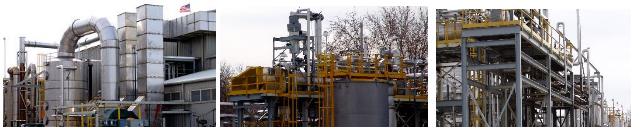
Figure 3. Three views of an HTL plant producing 3 million gallons per year of diesel fuel
